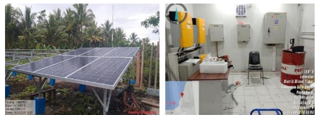
Fig. 6. 10 kWh Audam PV System
