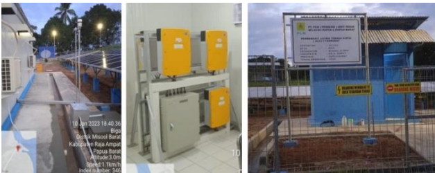
Fig. 9. 30 kWh Iwol PV System
