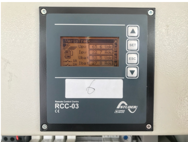
Figure 12. Local Monitoring Results with RCC-03 in Off-Grid Mode
