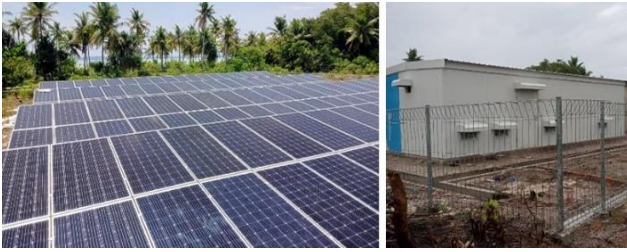
Fig. 8. 40 kWh Mutus PV System
