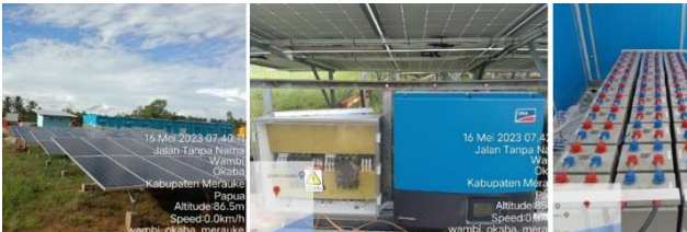
Fig. 10. 120 kWh Wambi PV System
